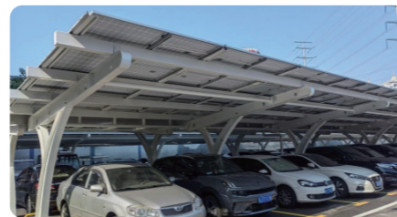
Waterproof PV carport
